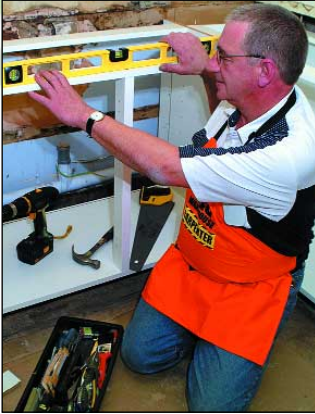
Dukeries during: B&Q fitter Clive Taylor installs the new units in his free time.
